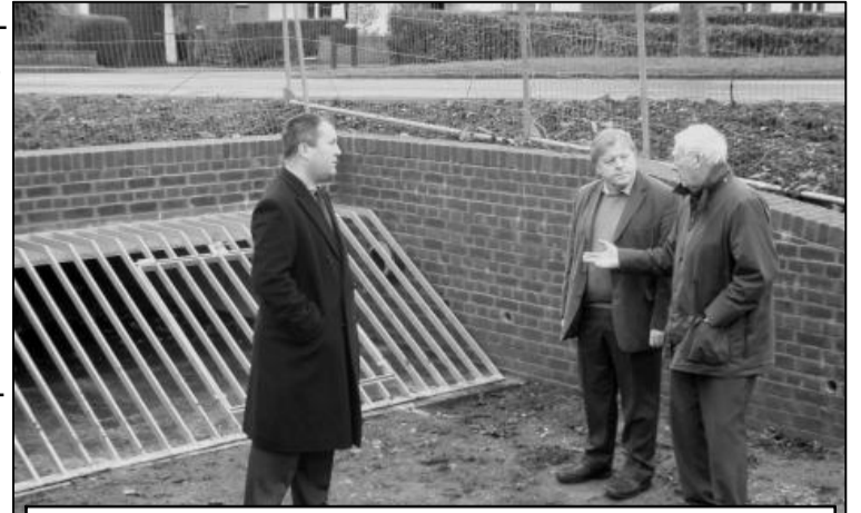
Cllr Martin Vye (right) shows the new Valley Road culvert in Barham to Parliamentary Spokesman Guy Voizey and Nigel Whitburn
